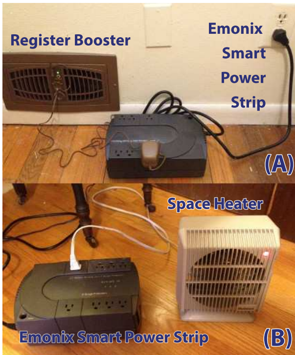
Figure 4: Photographs of our control equipment. (a) A register booster fan is controlled using an Emonix smart power strip by an off-site controller. (b) An Emonix network-connected power strip controls a space heater that provides additional heat in rooms that are too cold during the winter months.
